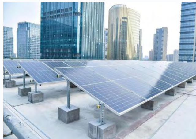
佛山数据中心“光伏+储能”项目 "Photovoltaic + energy storage" technology in Foshan Data Center
